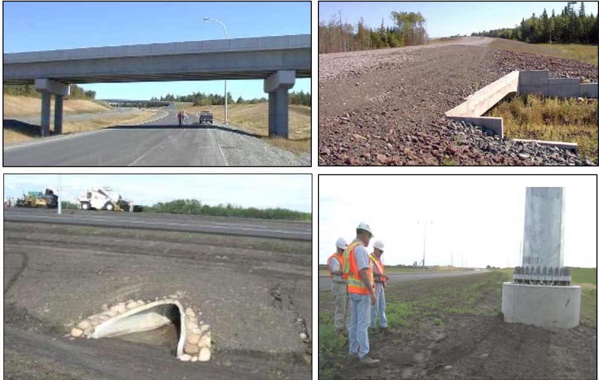
Figure 1: Examples of Hazards Placed at Minimum Clear Zone Offsets
