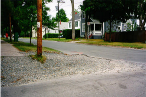
Photo 1. Unsigned construction at intersection
