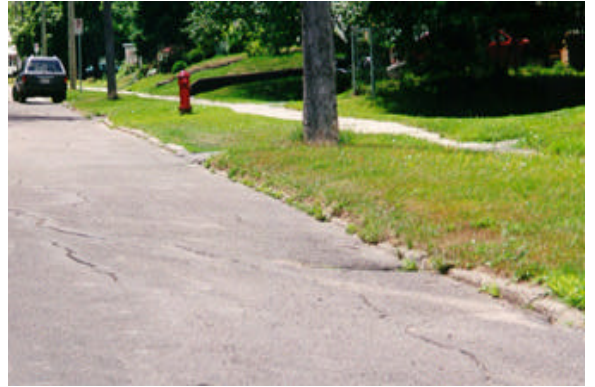
Photo 2. Curbs in disrepair
