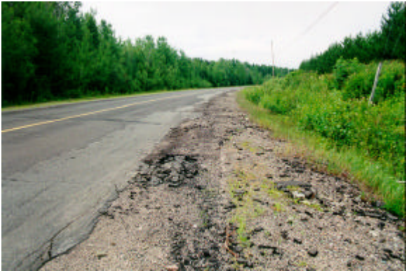
Photo 3. Ravelled pavement edge
