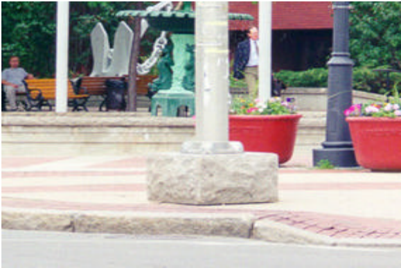
Photo 21. Pole with breakaway support on granite foundation
