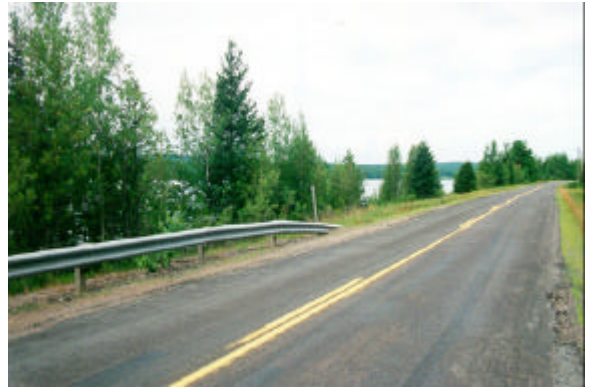
Photo 10. Inadequate coverage of guiderail
