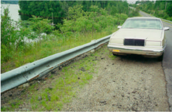
Photo 7. Guiderail too low
