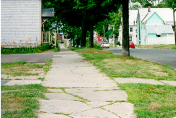
Photo 7. Poor sidewalk condition
