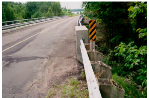
Photo 12. Guiderail not flush with bridge endpost
