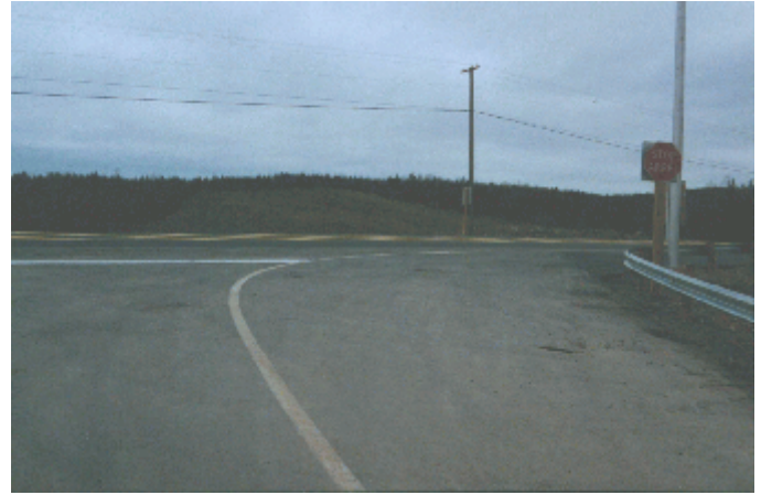
Photo 2: Excessive offset to stop sign (Route 25) off-ramp.
