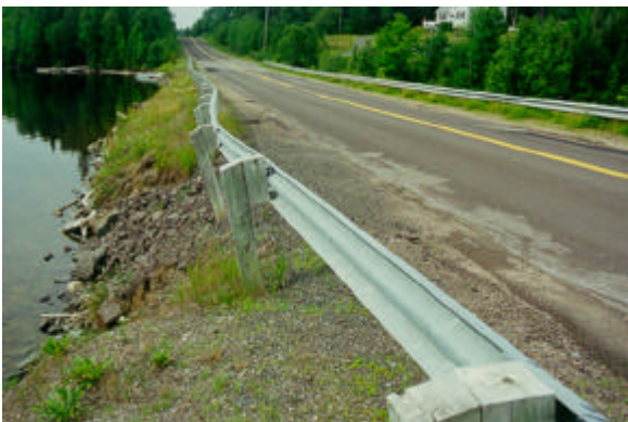
Photo 11. Washed out shoulder
