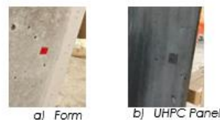
Figure 1: Surface Material Defect
