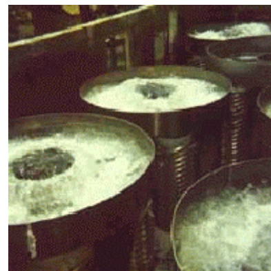
2: Packed columns used for H_2S scrubbing
