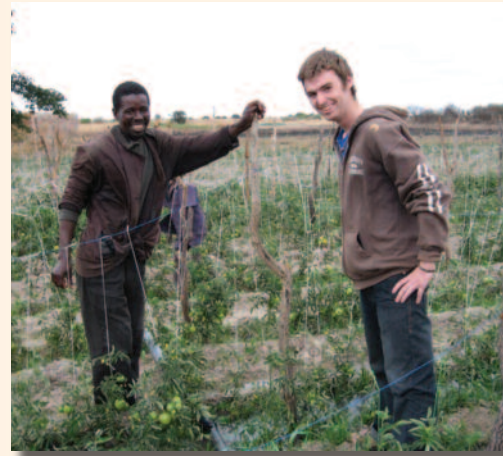
UNB student Brian Magee and his friend Robert Sakala lay an irrigation pipe in Zambia.
